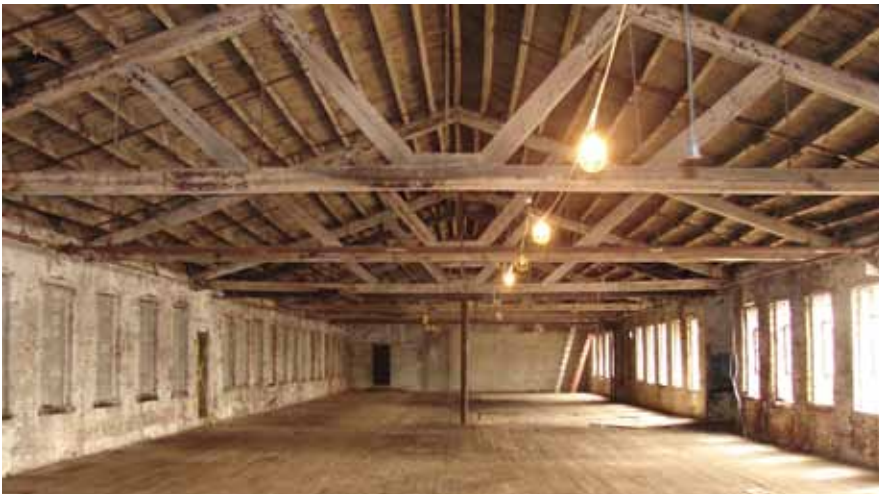
Figure 2: Lacking construction documents, visual inspection and detail field measurement were the primary means used to assess the buildings.
